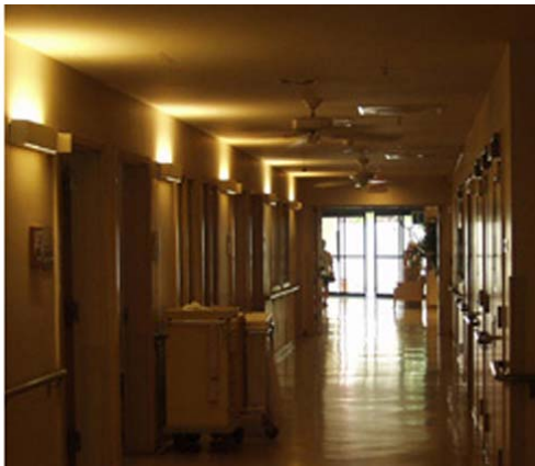
Figure I: An example of lighting problems a) glare from doors at the end of the corridor, b) uneven lighting, and c) low light levels.
